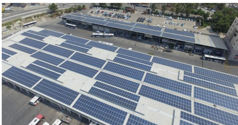
Fig. 2. The solar power plant, consisting of 3,680 photovoltaic (PV) panels, installed on the roof of ESHOT's workshop
